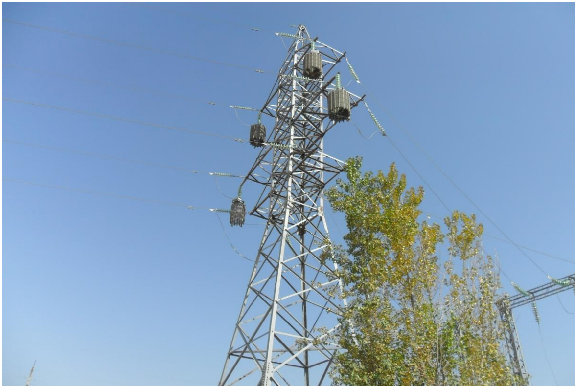
1.2 - rasm. Kuchlanishi 110 kV li havo liniyasi
