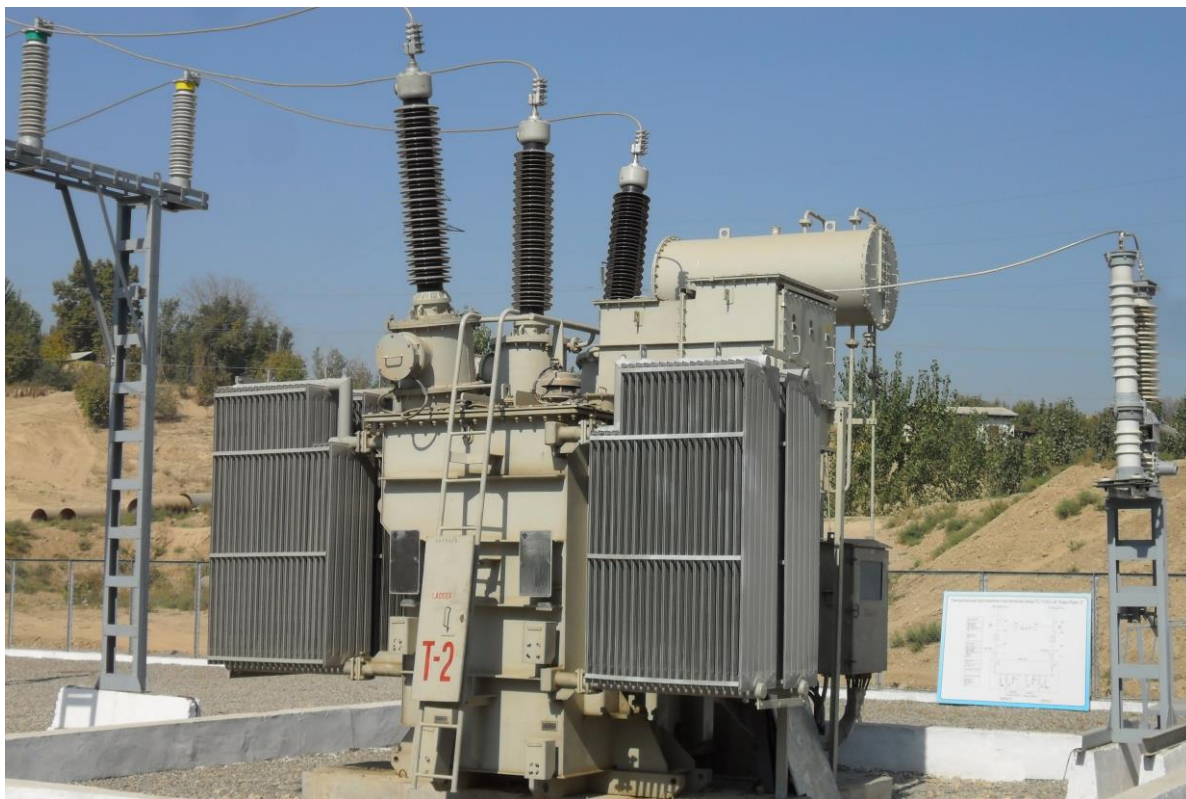
1.1 – rasm. Kuchlanishi 110/10 kV li quvvati 16 000 KVA li moy transformatorli podstansiya
