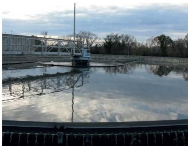
Figure 7.8 A circular primary clarifier.
